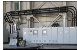
Cables (Top) vs. IBP (Bottom)
